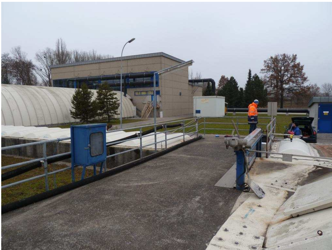
Figure 30: Installation site of the inflow measurement devices to the primary clarifiers
