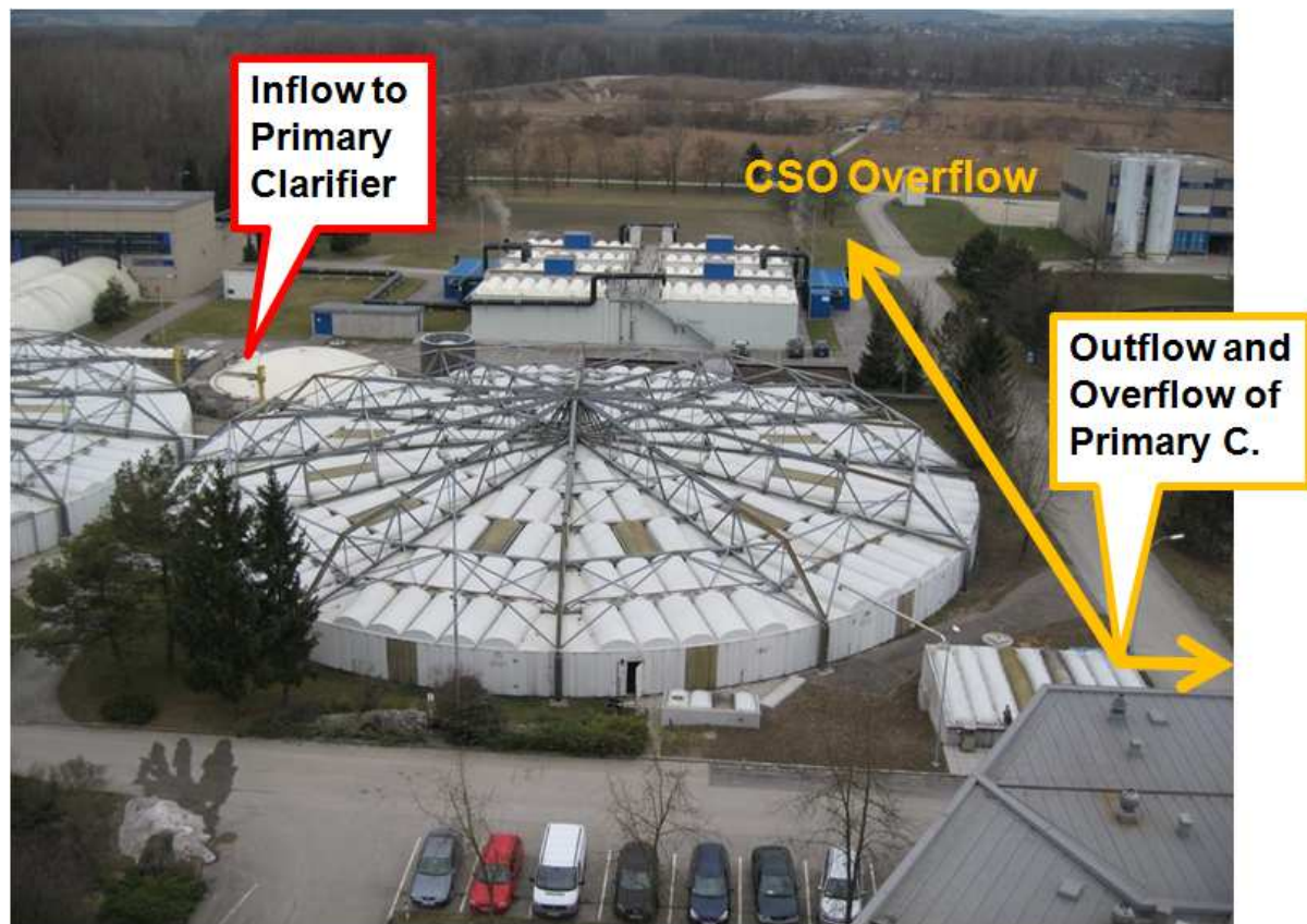
Figure 29: Photos of primary clarifiers indicating inflow, outflow and overflow situation
