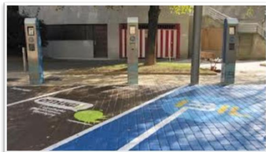
Figure 4.2.3.2 Emugi Charging station
