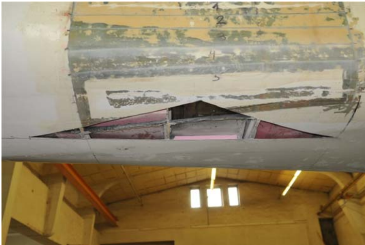
Figure 10: Cruise Vessel C1, Bottom Damage from #183 to #243
