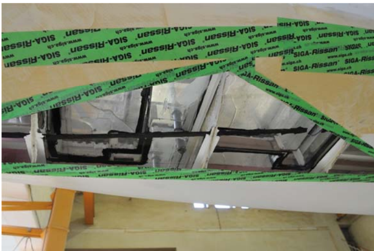
Figure 12: Cruise Vessel C2, Bottom Damage from #228 to #305
