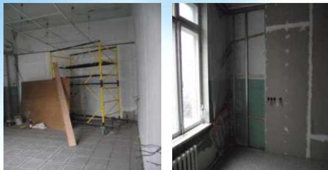
Rooms of Joint SES Laboratory before repairs
