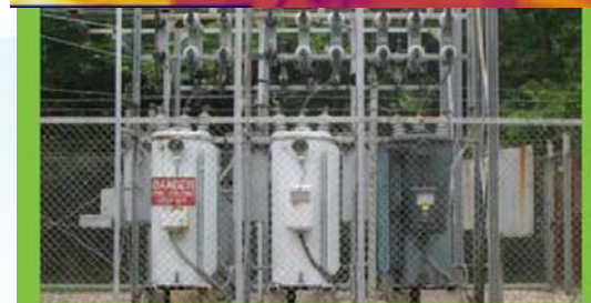
Examine transformers, comparing similar connections under similar loads.
