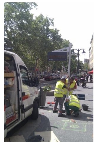
Figure 18 Installation in Lyon
