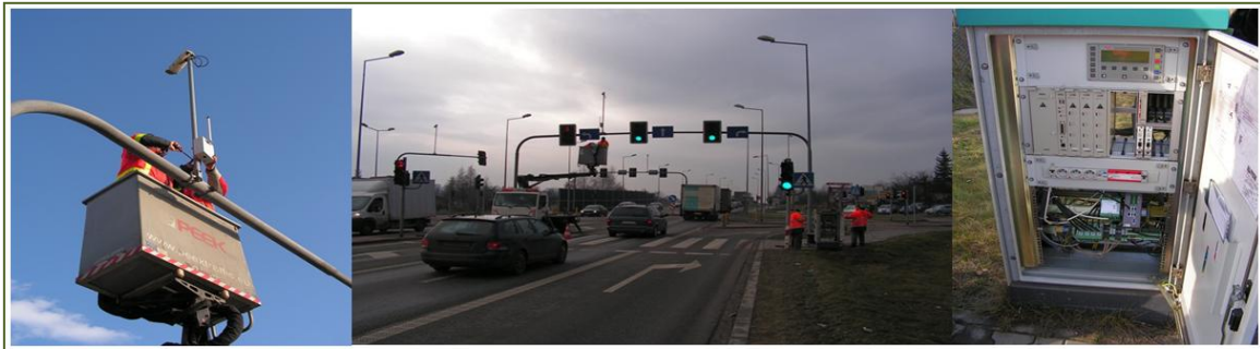
Figure 6 Road side installations of FREILOT Energy Efficient Intersection Control in Krakow
