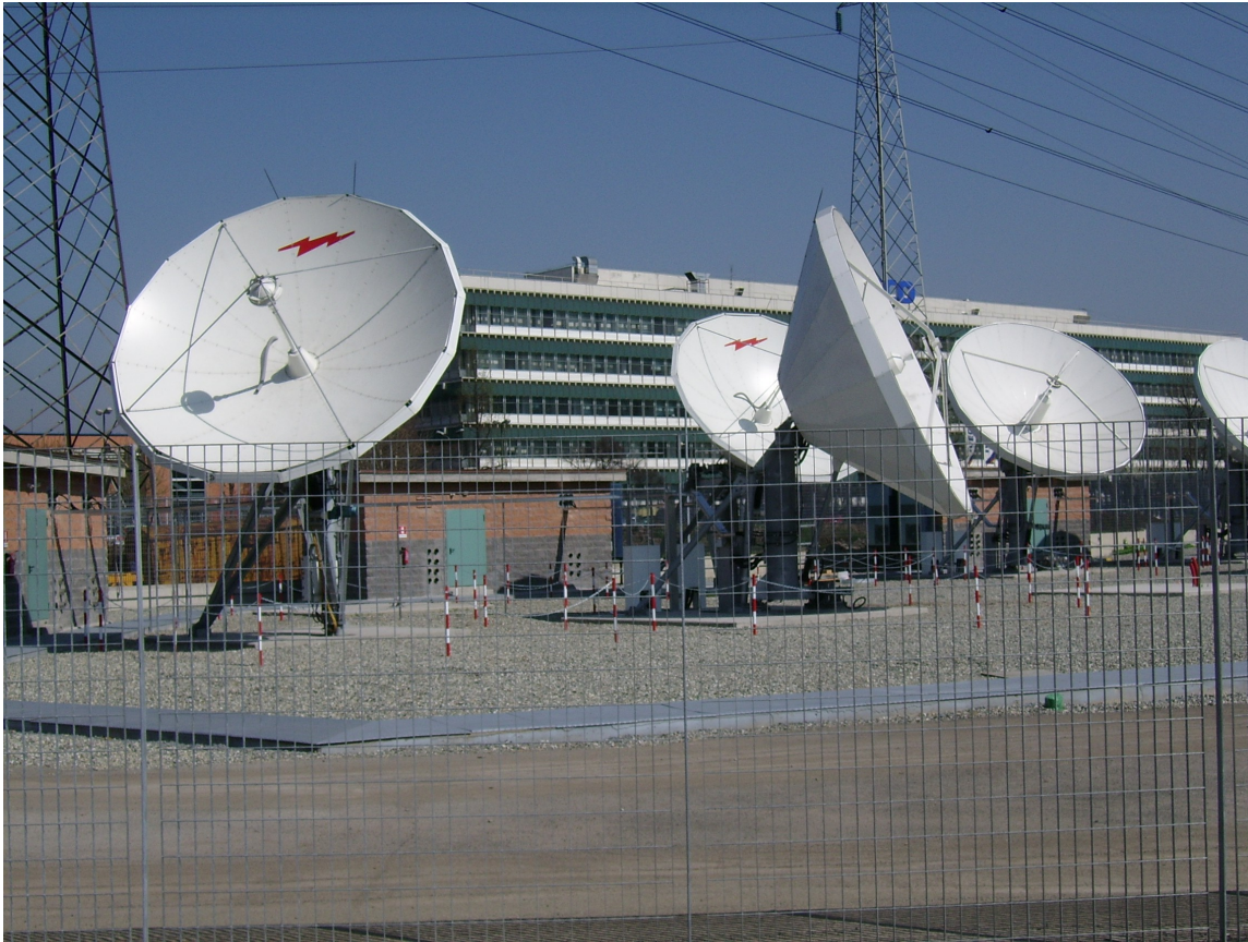
Figure 8: Example of antennas in a teleport
