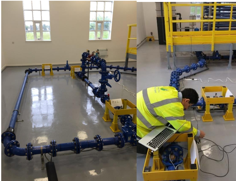
Figure 6: DCWW Test Rig
