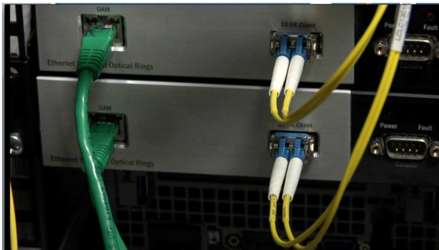
Figure 10: 10Gbit XFPs connecting Optical Switch to OPST nodes
