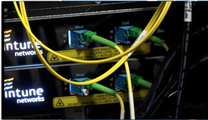
Figure 9: OPST nodes installed at PrimeTel HQ Data Centre
