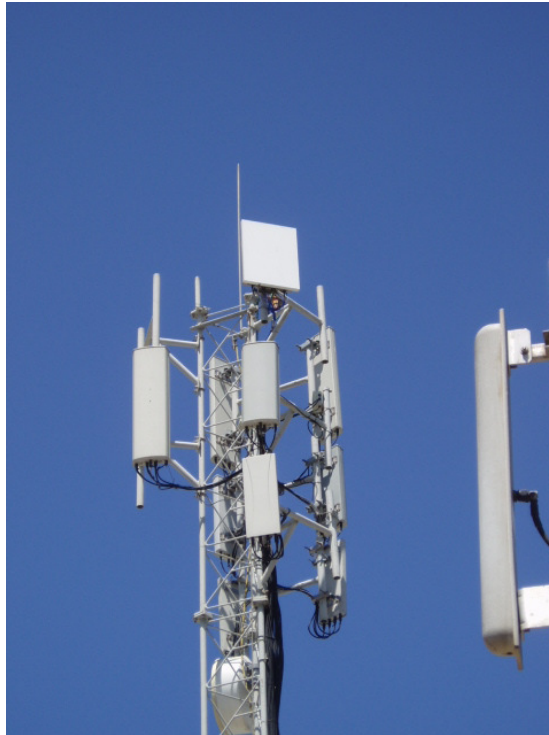
Figure 7-5: HBS antenna on top of mast during live test at Alvarion's premises, Tel Aviv.
