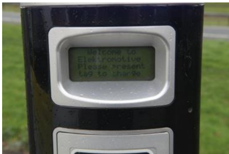
Figure 91: Available and functioning charge point
