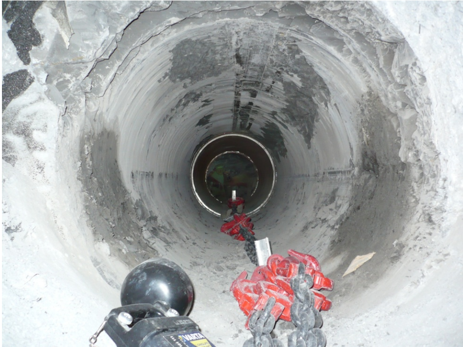
Figure 2: Front casing element blocked in the ground (Casing elements 2 and 3 have already been withdrawn)
