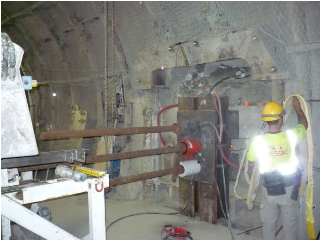
Figure 3: Equipment put in place for the withdrawal of the front casing element
