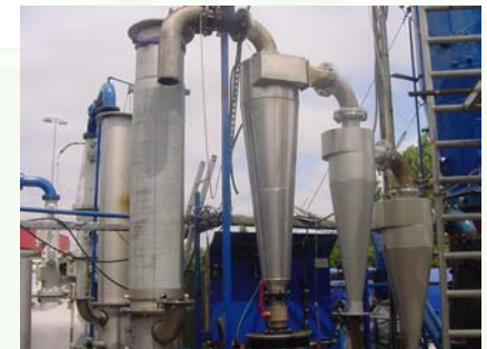
New organic scrubber
