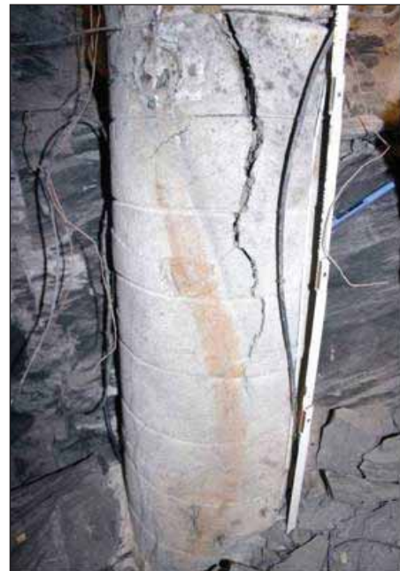
Figure 5.2: Bentonite buffer with dry crack in 330-direction, blocks 12 to 5, depth 5.80-6.60 m, sensor FB00_05.80 at block 12, brownish coloration coming from the sensor due to corrosion during hydration.
