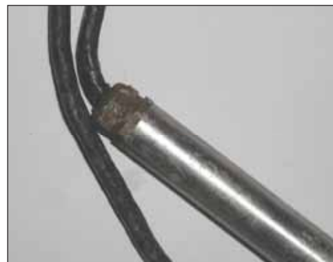
Figure 4.11: Corrosion in the metallic cable gland of a relative-humidity sensor.
