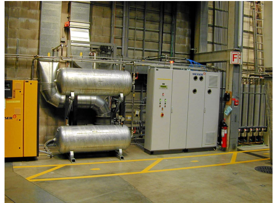
Fig.1: LowOx-unit with compressor, puffer tanks, control racks and membrane unit (from left to right)
