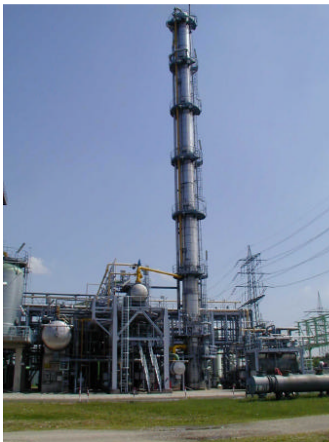
Figure 5: Propane/propylene splitter (Targor plant)
