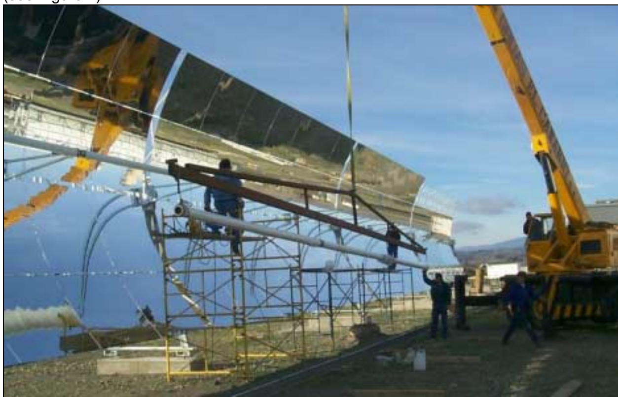
Figure 2 EURO Trough prototype installation at the PSA
