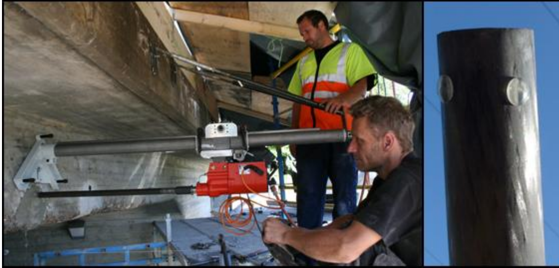
Figure 6. Left: Drilling 9 m long 38 mm diameter holes for strengthening the bottom slab of a concrete railway trough bridge using 4 mm wall thickness 32 mm diameter CFRP tubes. Right: A close up view of the tube end.
