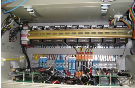
Figure 10: Control system module
