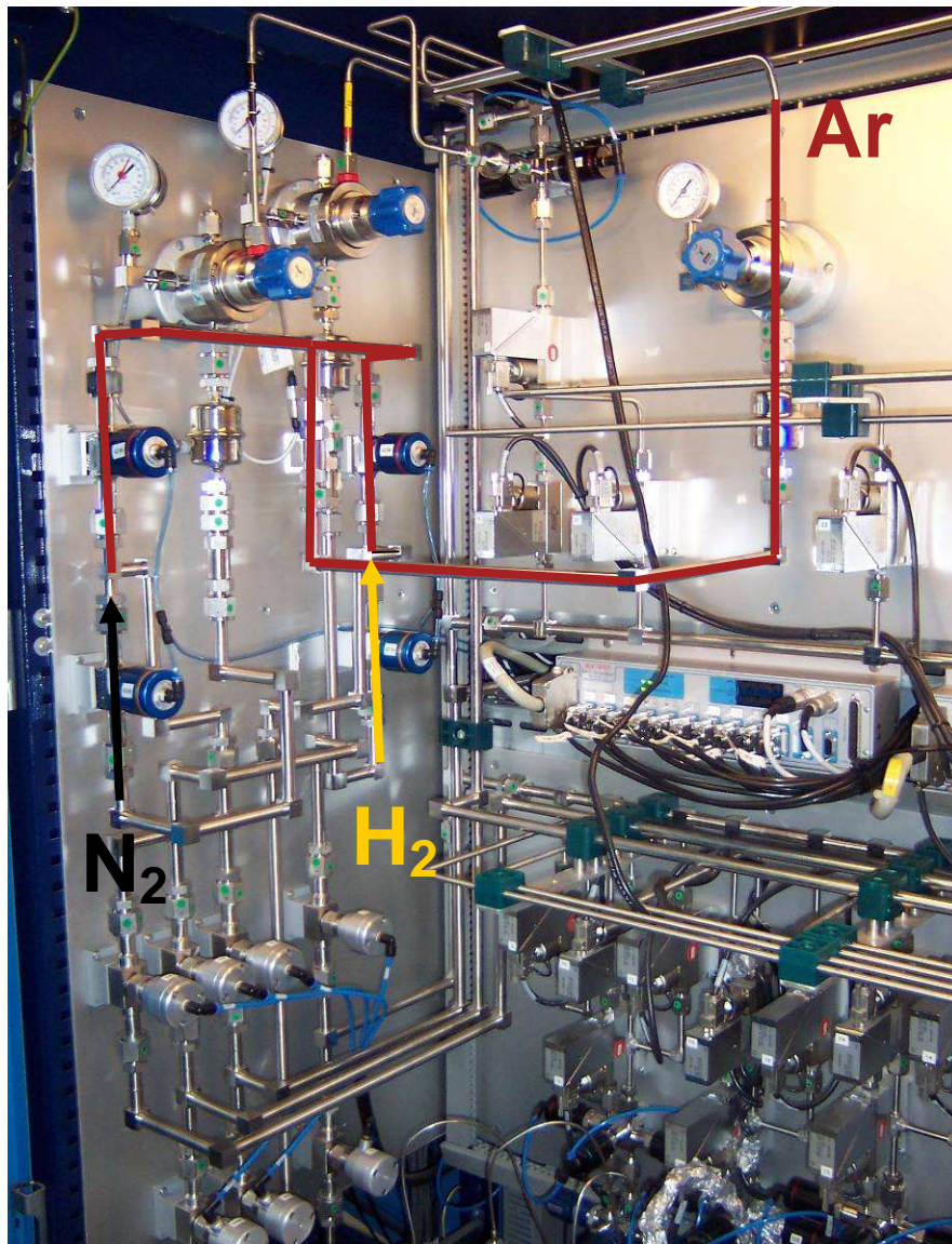
Fig. 24: Installation of third carrier gas line (Ar) into the AIX200/4RF-S reactor in Montpellier. The three carrier gases can be switched individually or can be mixed.
