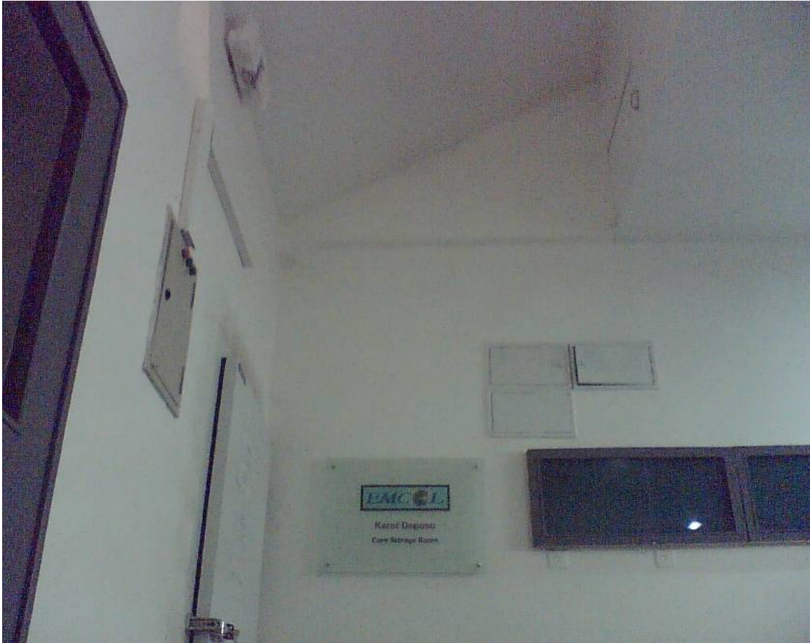
Fig. 16. Cold Core Storage Room fitted with temperature and humidity display unit and alarm.
