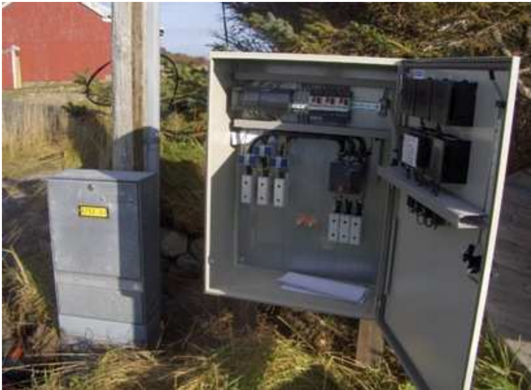
Figure 24 – Grid connection point
