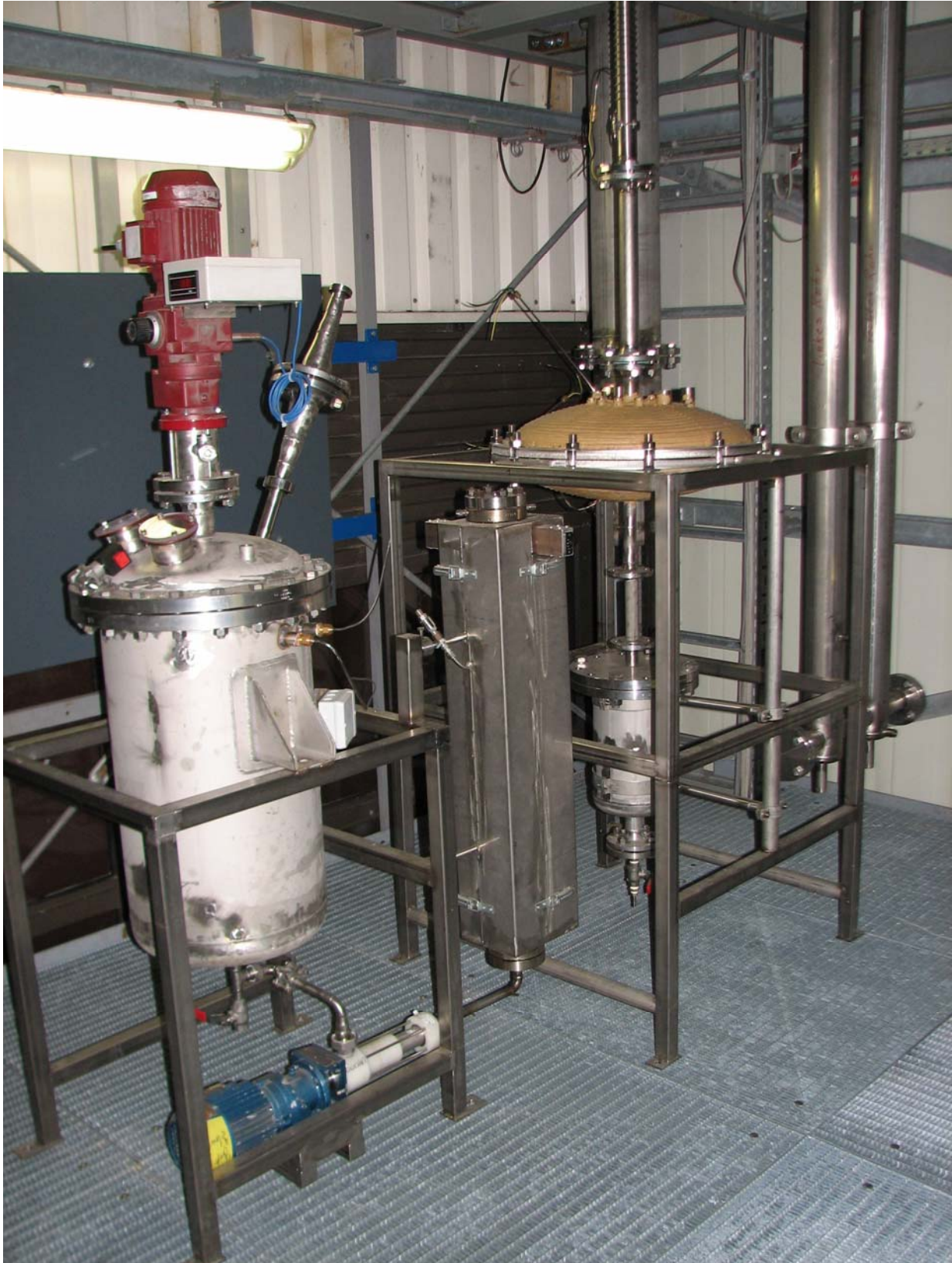
Figure 14: Part of the Oberhausen sts-plant. The remaining part is located in the upper floor.
