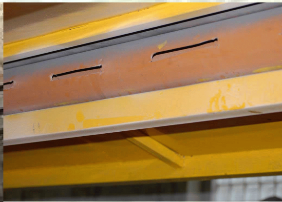
Ventilation air intake installed on pipe manufacturing line
