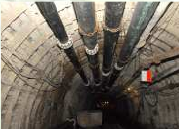
Pipes are used for ducts in underground hard coal mine – in severe mechanical and explosive environment
