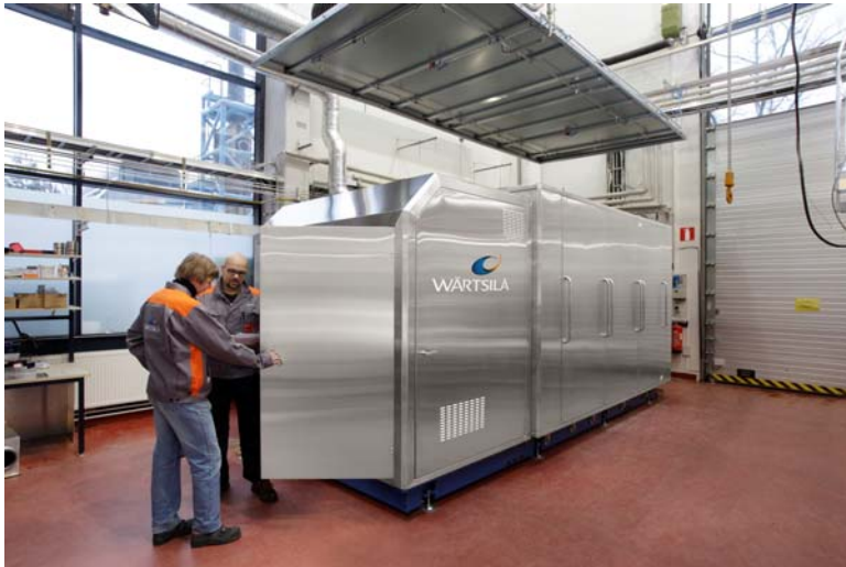
Figure 8.1. WFC50 installed at the test site.
