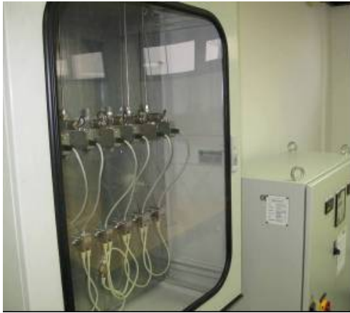
Figure 6.32. Mass-flow controllers and ventilated cabinet.
