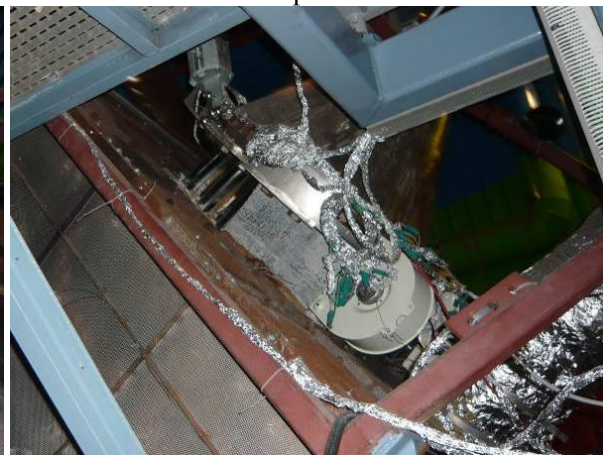
Figure 63 Additionally installed cooling fans
