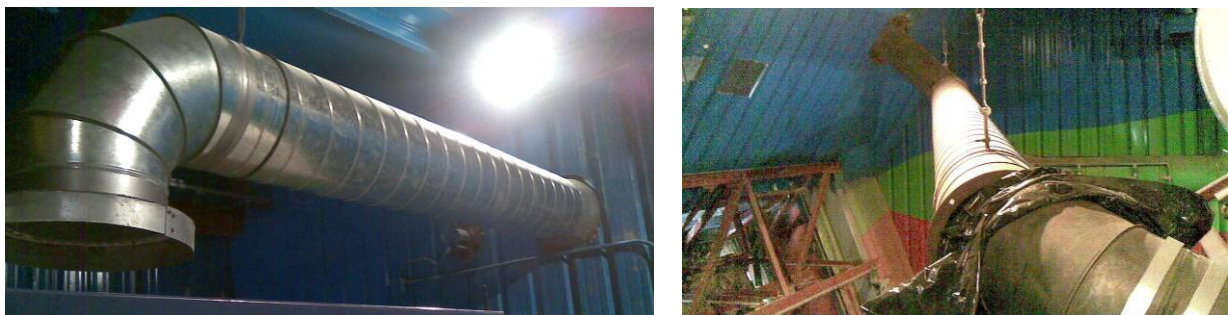
Figure 45 Air Inlet and exhaust gas piping
