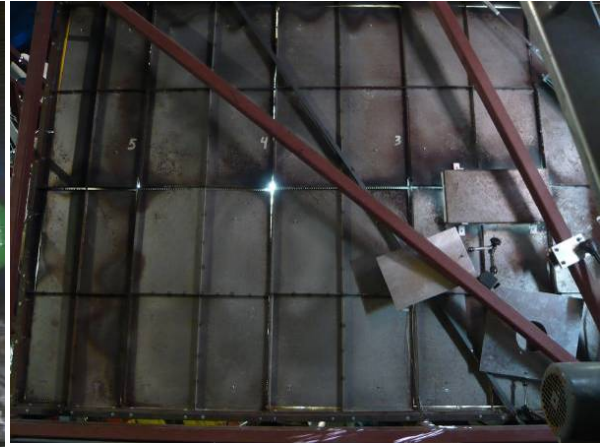
Figure 61 Gaps in cavity wall after approx. 45 hours of operation
