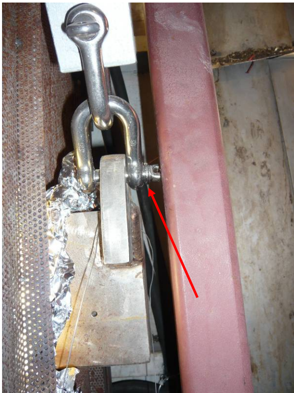
Figure 67 Shackle of receiver suspension touching the frame structure
