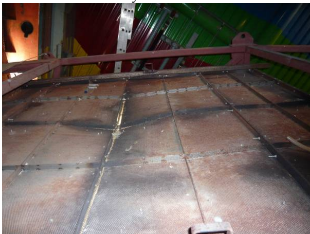
Figure 62 Top of cavity with overheated metal sheet
