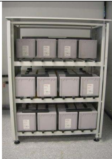
Figure 3 – Lead acid battery
