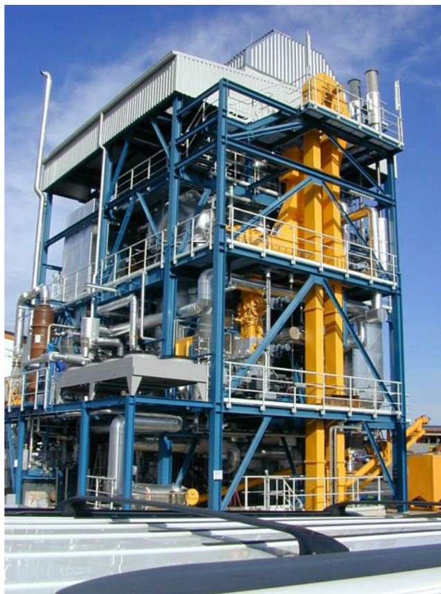
Figure 3: 8 MWth biomass CHP plant Güssing
