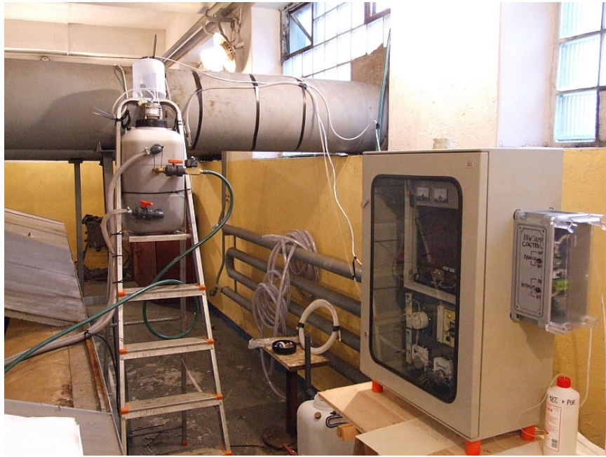
Fig. 17 The METELCAD monitor setup at the Bohumin site.
