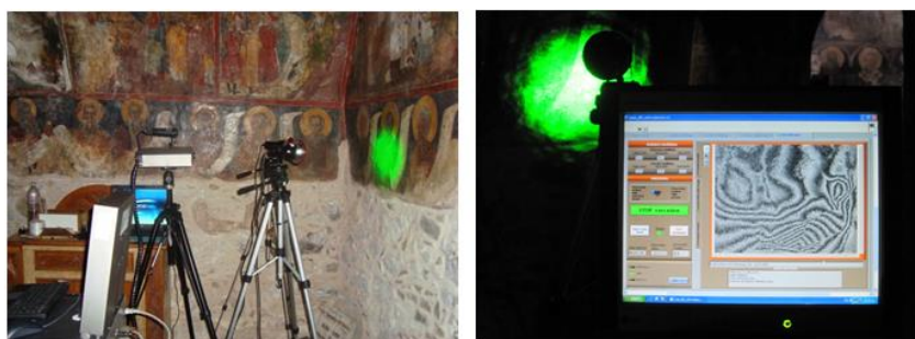
Fig. 3.4.6 On-field defect mapping of wall paintings in Museum church with real time raw data visualizing highly structured subsurface interconnection among crack and lateral detachments
