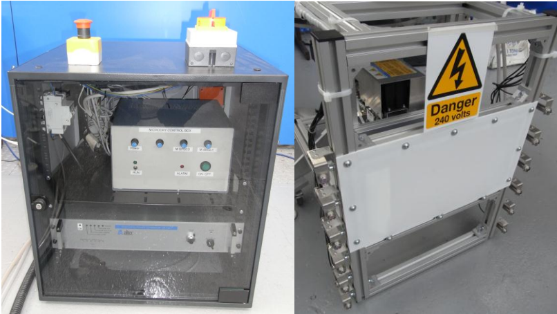
Control Box & PLC in Control Cabine & Front End of Microdry Unit with Infra-Red Sensor
