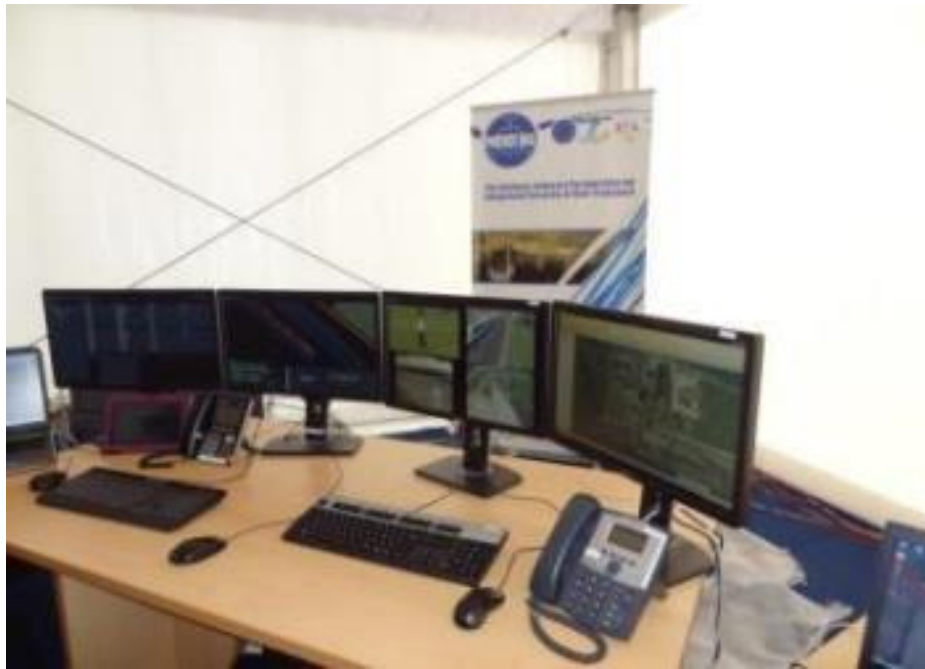
Figure 43: The Control Room
