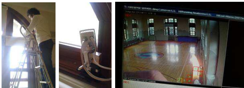
Figure 24: Installation of camera in Dodge Hall and screenshot from internal camera view
