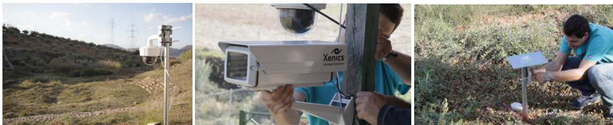
Figure 22: Optical PTZ camera, IR camera and WSN nodes installed in Kabeirion.
