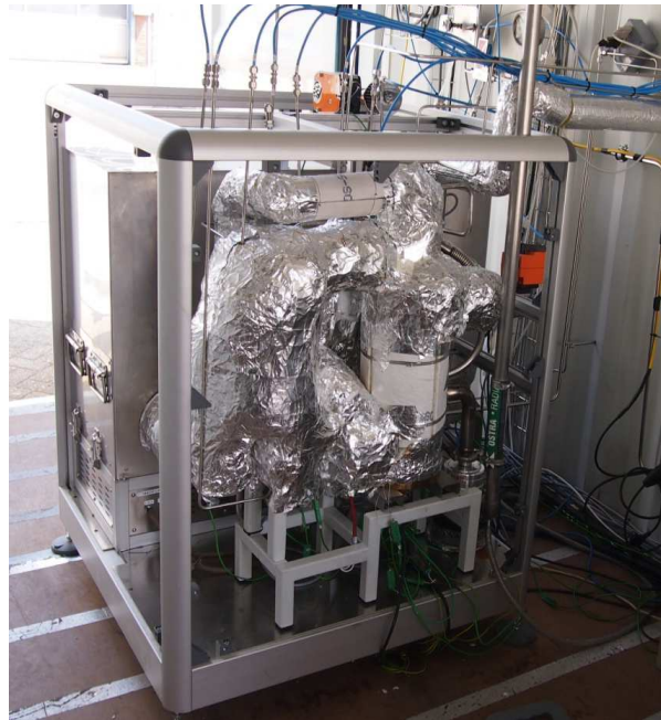
Figure 27: LOTUS system: reformer side, insulated
