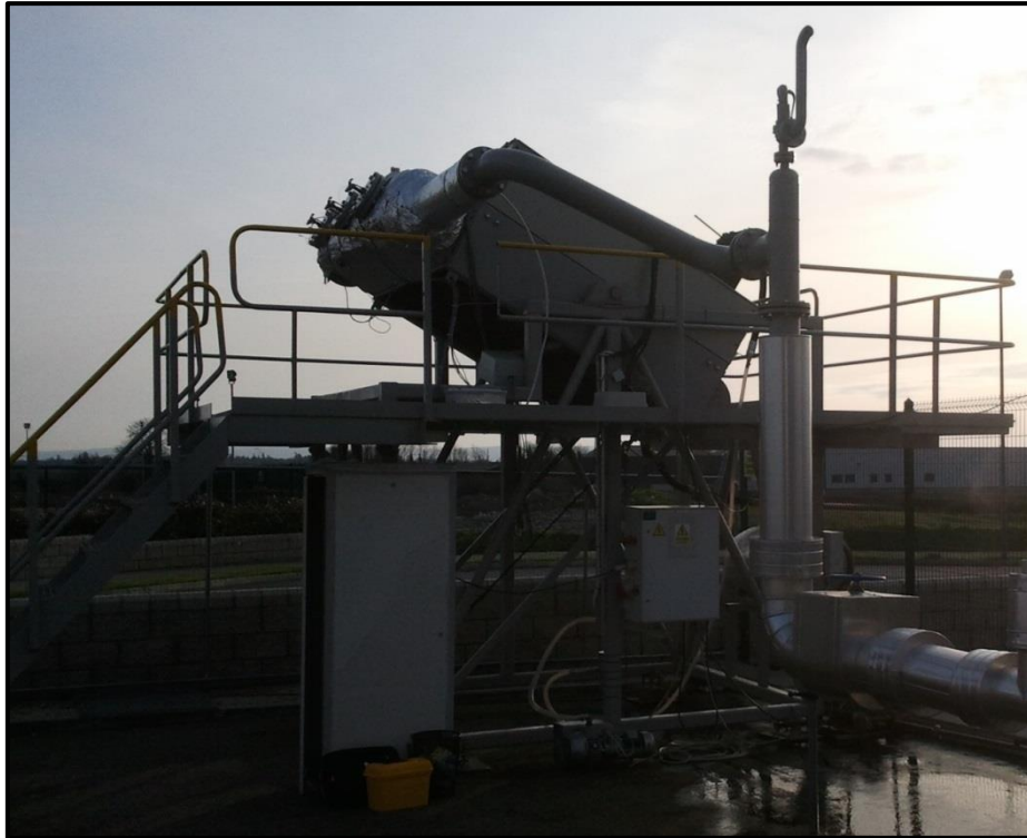
Figure 9: Operational MACC prototype on-site
