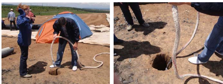
Figure 3.51: Albota Landfill Chemical Sensor Installation
