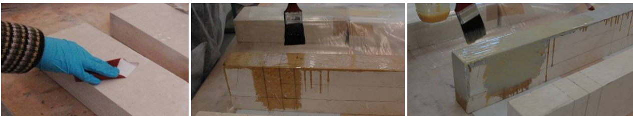
Figure 3.45: Preparation of the substratum (left), Application of a first layer (middle), Application of an epoxy resin layer (right)
