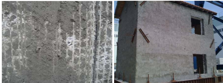
Figure 3.53: Eucentre-Polymast full-cover textile reinforcement: mortar + textile as they look like when applied to the wall (left); the building full cover after some days (right)
