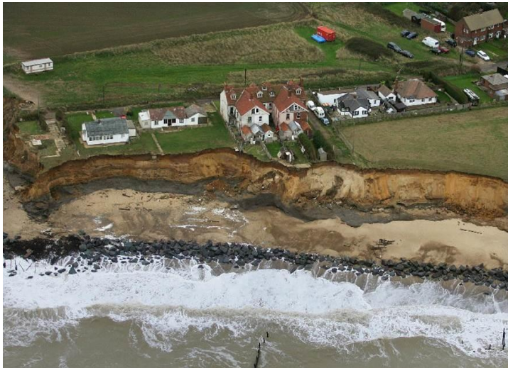
Coastal damage during a flood, courtesy Angela Scott, Environment Agency
