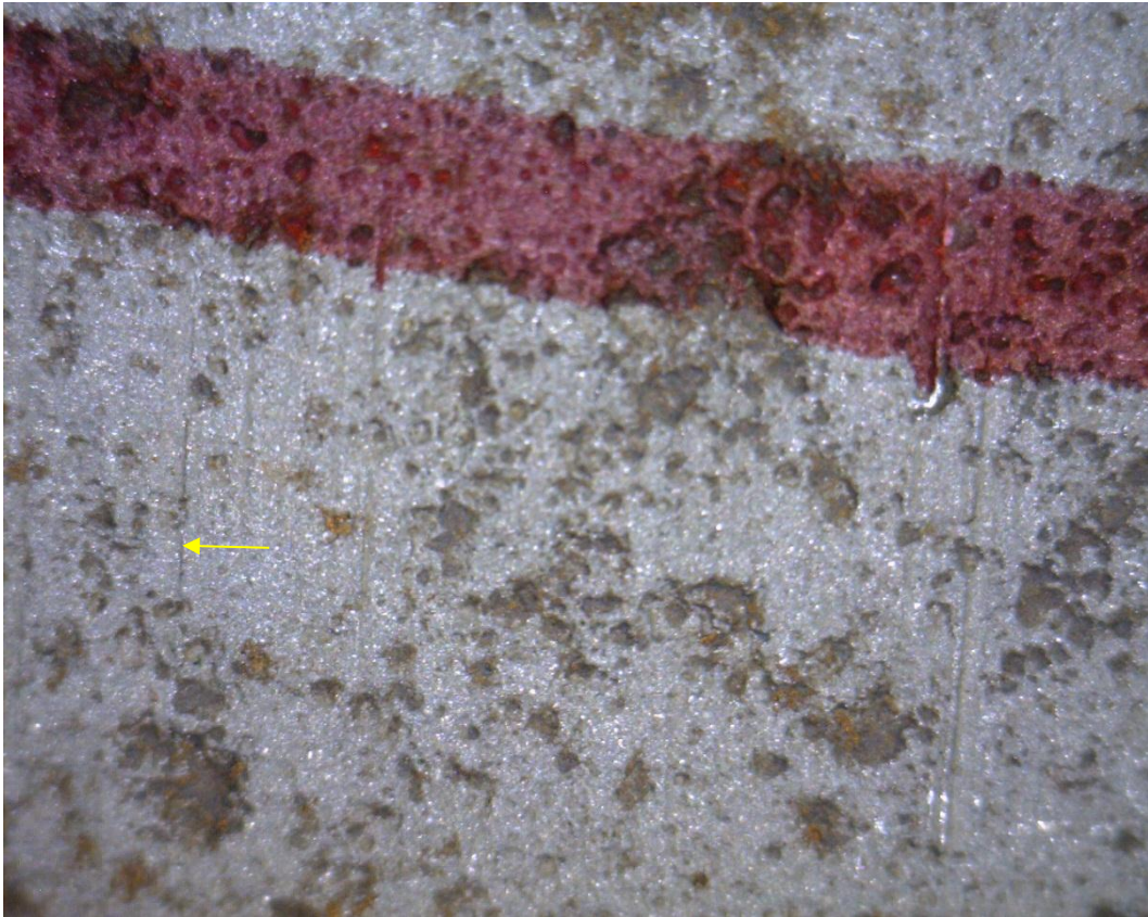
Figure 17 Example of Cracks Detected
