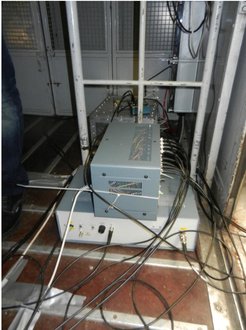
Figure 22: Installation of the supporting electronics. The EMAT pulse generator and amplifiers are in the foreground while the pneumatic and electronic controls for the deployment frame are towards the back of the compartment.
