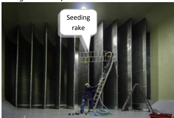
Figure 3 Installation of the seeding rake at the final turning vanes just before the contraction section.
