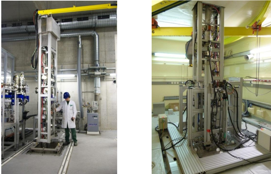
Figure 13: (Left) Upper level of the accelerator during beam line handling: the vertical line is being inserted in the reactor bunker while the magnet is retracted. (Right) Vertical beam line inserted into the reactor core.
