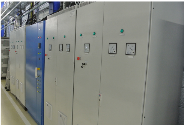
Power Electronics Cabinets
