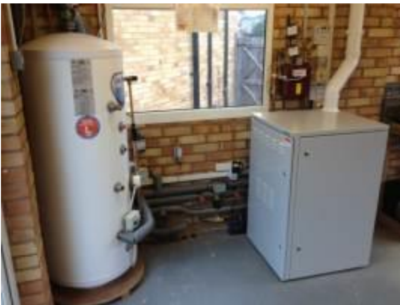
A typical installation in a UK garage
