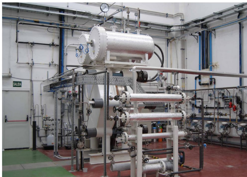
Figure 14 Picture of the electrolyser of IHT at FHA facilities
