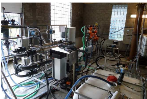
Figure 18: Nanofiltration pilot plant with HCNF1 membranes at VMW
