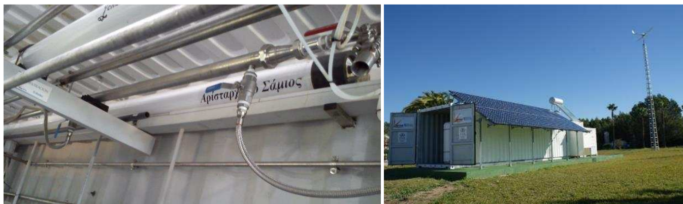
Figure 17: Left, picture showing HCNF1 pressure vessel installed in ETAPERN plant substituting an original 4040 pressure vessel, right external view of the container of ETAPERN plant and PV and windmills units
