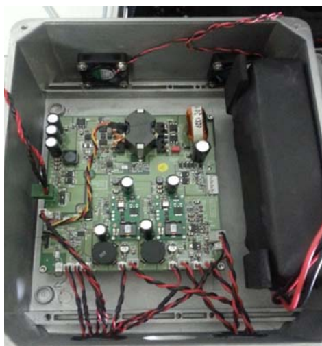
Figure 8: Battery system in its own housing.
