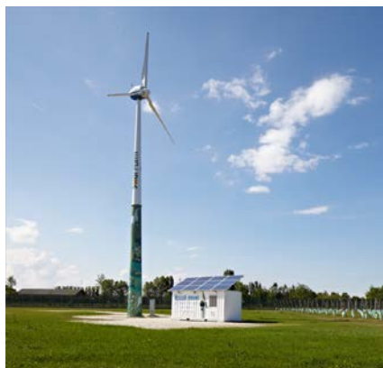
Fig. 28: 7 kW TRE wind turbine installed in a remote location.
