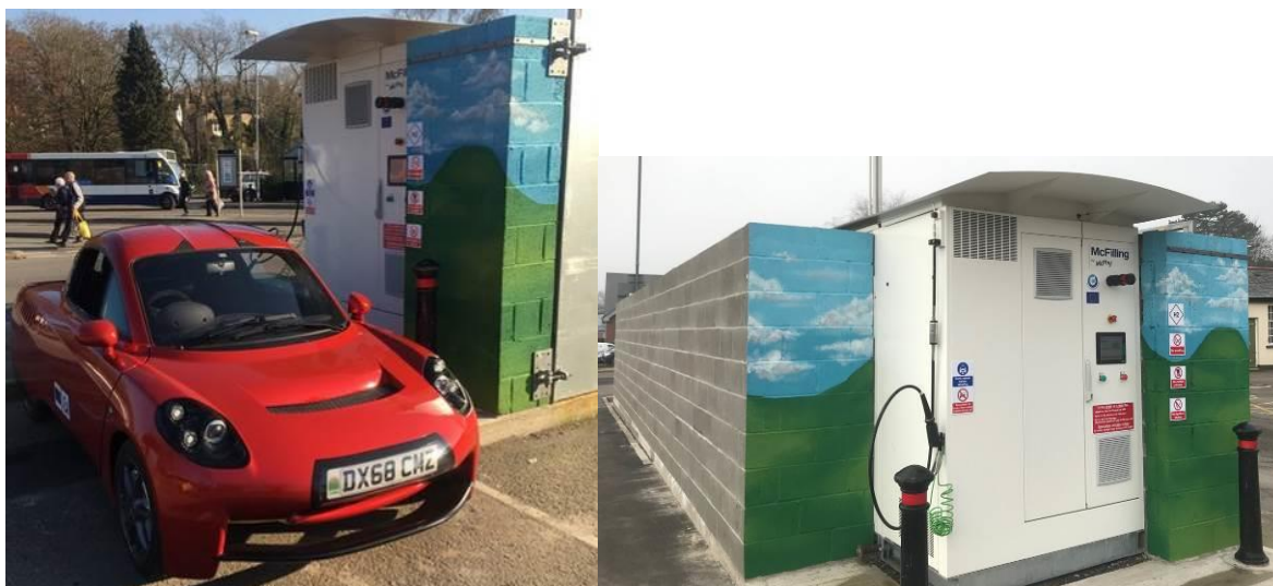
Figure 11 - Installed McPhy refueler in Abergavenny with Riversimple Rasa Beta vehicle
