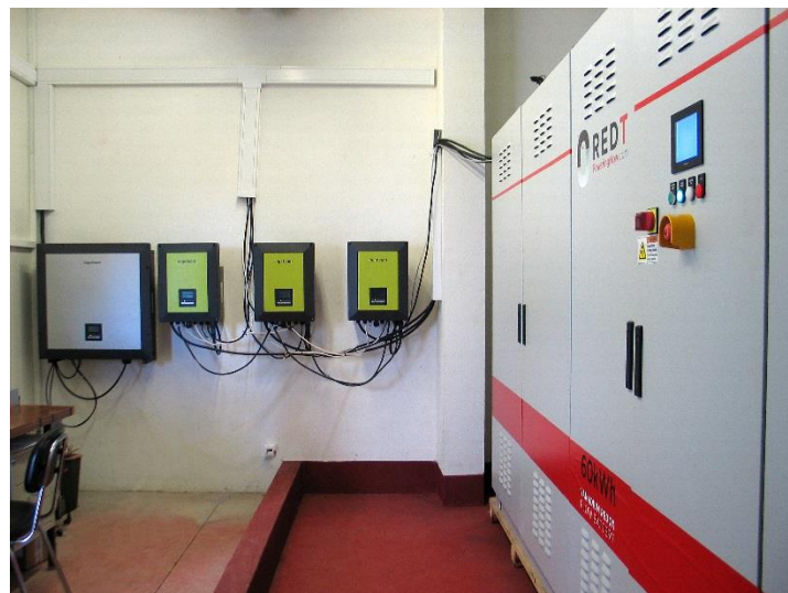
Figure 10. VRB system installed at Évora's university.
