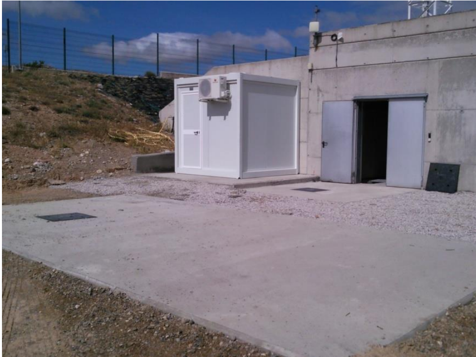
Figure 9. Lithium ion energy storage system installed at Tudela PV plant
