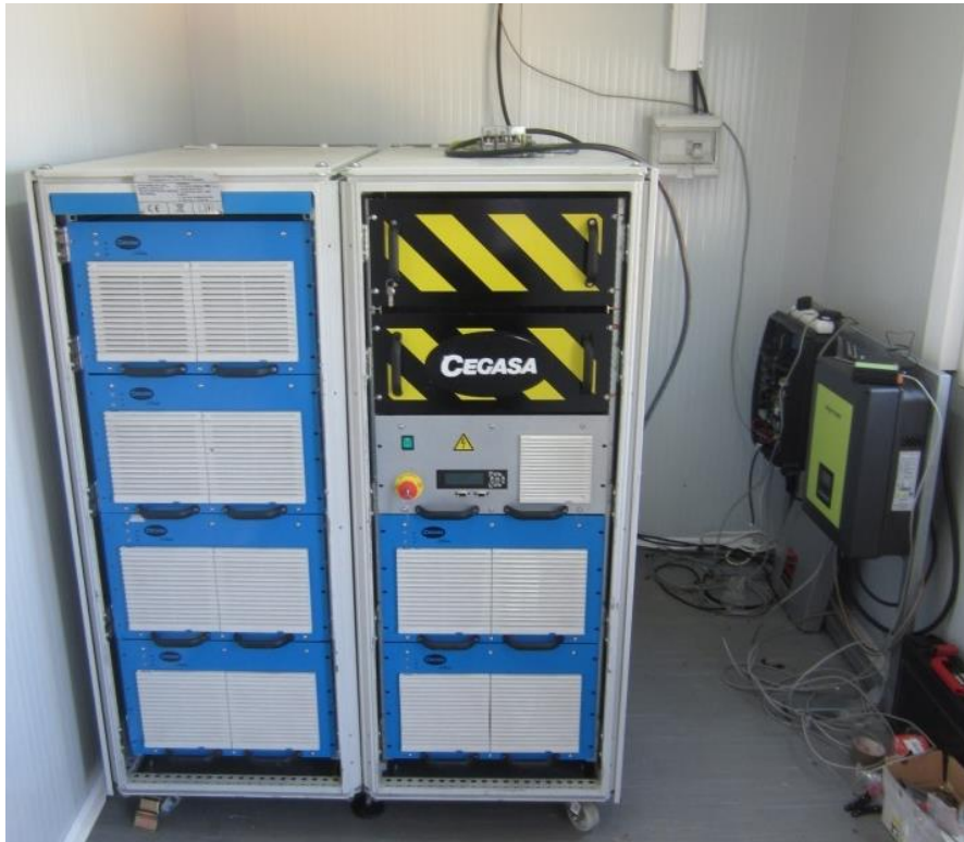
Figure 11. Li-ion demonstrator at University of Évora. Ingeteam's power inverters on the right and lithium-ion battery on the left.
