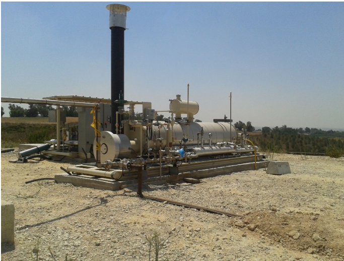
Figure 3: the heat exchanger
